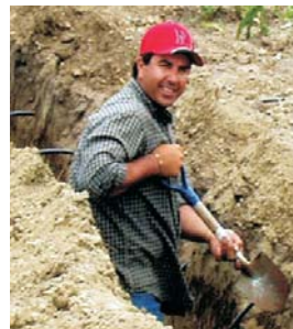
Dr. Irmak connects individual drip lines to the main lines. A total of 344 drip lines were connected.
