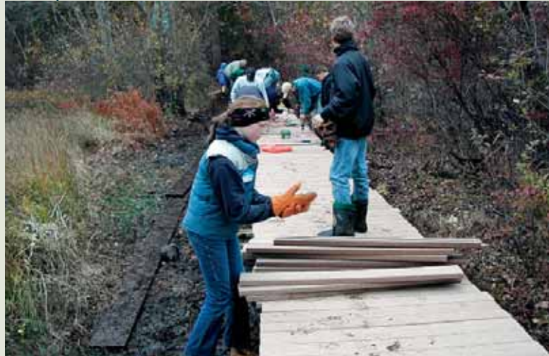
Volunteers with the Carlisle Trails Committee spent two days building a footbridge at Great Meadows NWR, MA. New improvements to the River Trail are giving refuge visitors better wildlife viewing opportunities through refuge wetlands. (Bert Willard)
