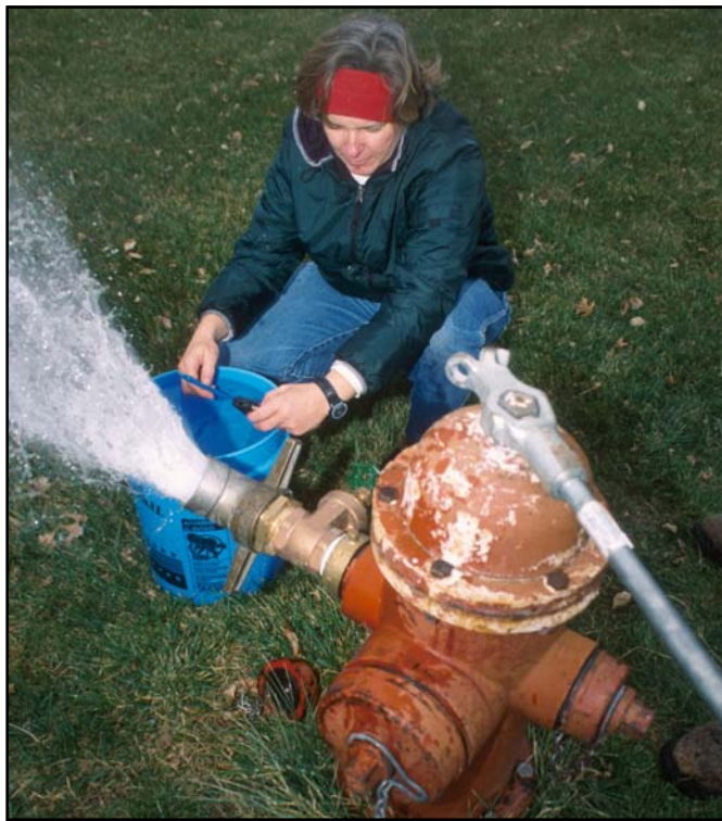
UNL School of Natural Resources project coordinator Lynne Klawer monitors pH and temperature during a water main flush at Stromsburg that is part of a project to help small communities find lower-cost ways to reduce or eliminate arsenic in drinking water (IANR photo: Brett Hampton).
