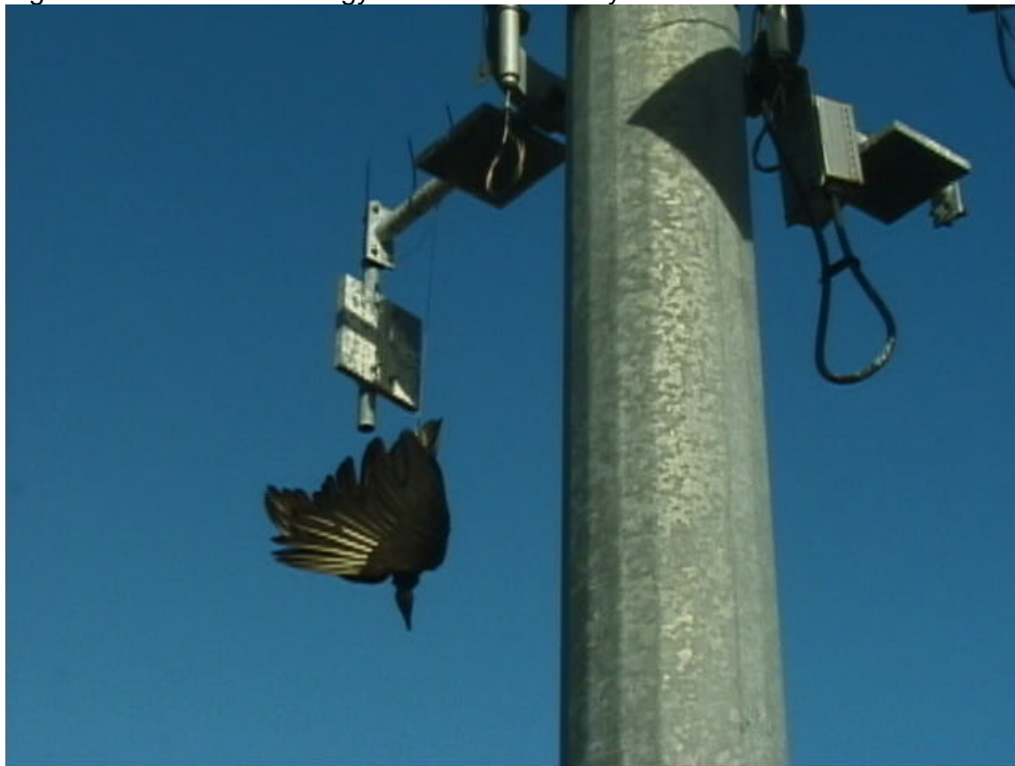
Figure 9. Black Vulture Effigy in Place on Fort Myers LLWAS Remote Station #5
