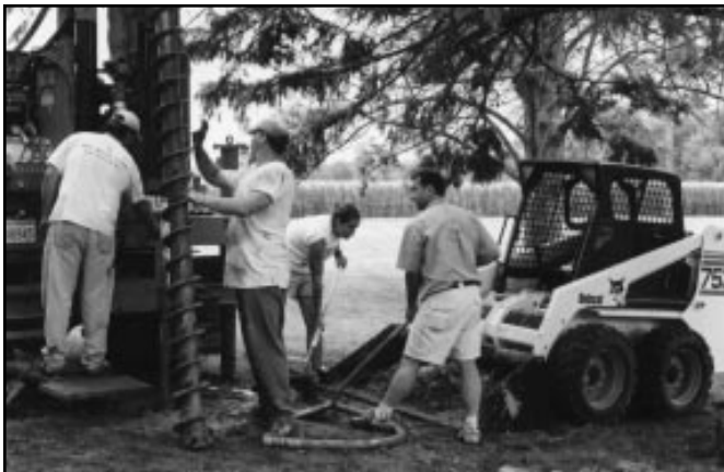
Staff from the UNL Water Sciences Laboratory work on building a daisy well denitrification system in southeast Nebraska (photo: Steve Ress).
