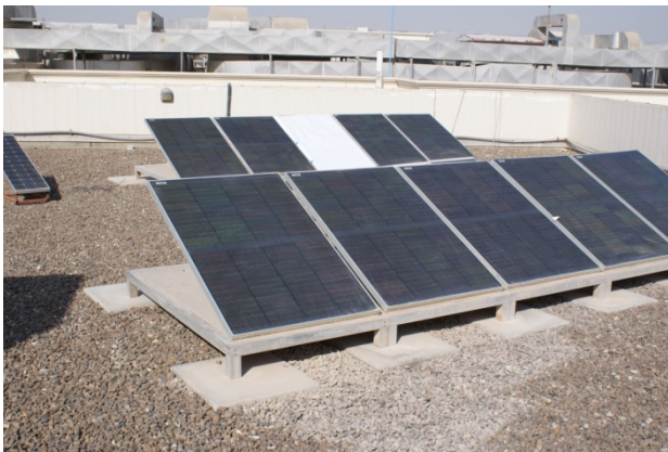
Figure 4: PV System in Petroleum Institute, UAE
