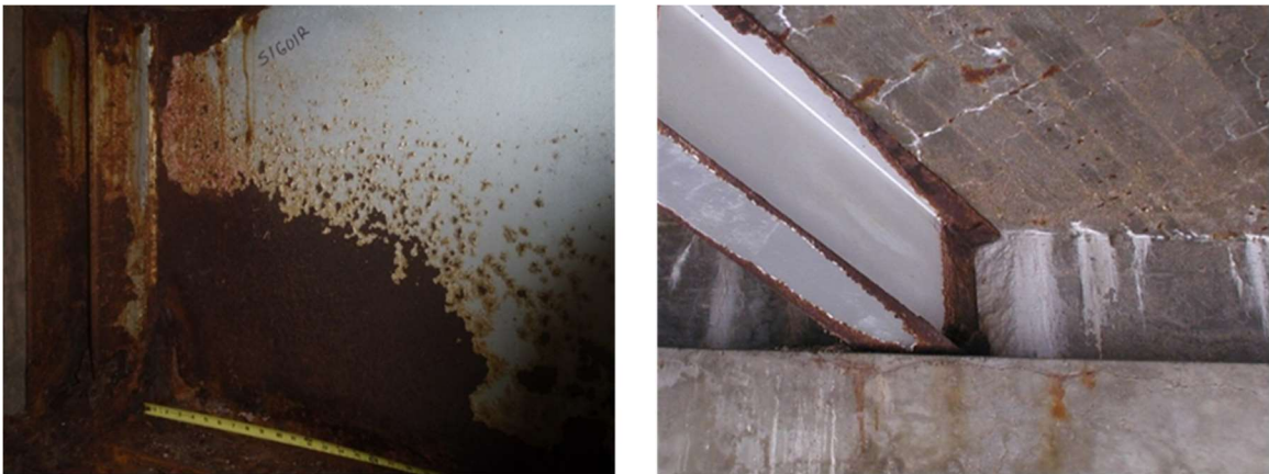
Figure 4.1 Deterioration pattern at girder ends
