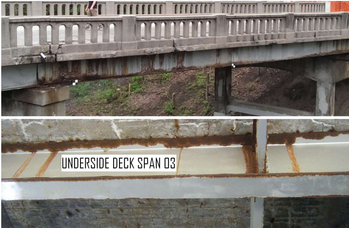
Figure 4.3 Deterioration pattern where entire section of girder is deteriorated
