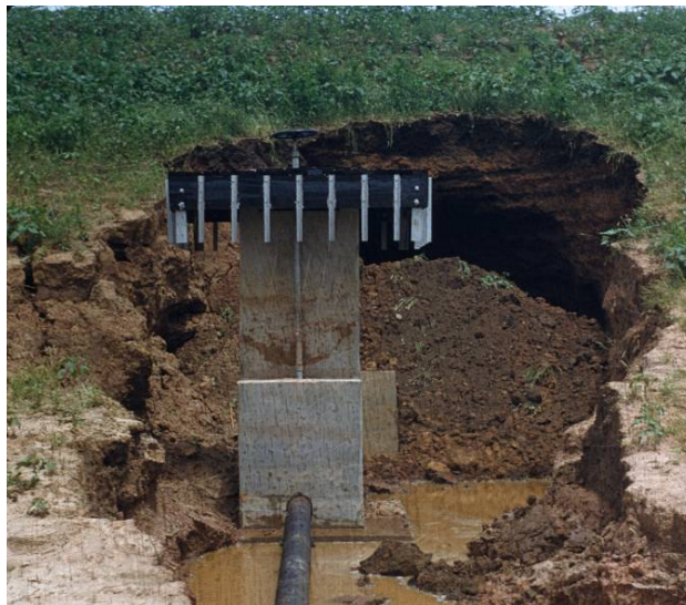
Figure 3. Typical small embankment failure resulting from hydraulic fracture of an embankment constructed of highly dispersive clays.
