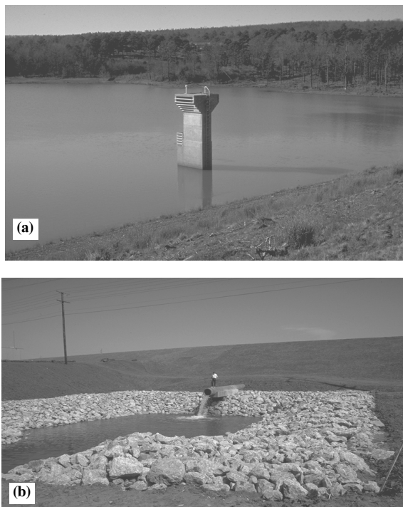
Figure 4. Components of the closed-conduit spillway: (a) trash rack and drop inlet tower, and (b) cantilevered outlet and plunge basin.
