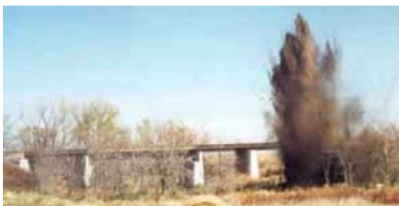
Figure 6 .Use of explosives to remove beaver dam and control potential undermining of a trsettle(Photo Credit: Ronald Fryda).
