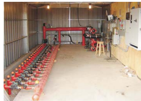
The SDI control unit includes: irrigation controller, variable speed controller, water and fertilizer flowmeters, chemical injection pump, along with numerous filters and valves.
