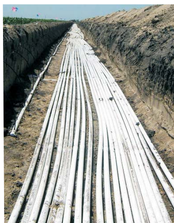
About 5 miles of 3-inch pvc pipe were installed to deliver variable rates of water to twenty treatments with three replications each.
