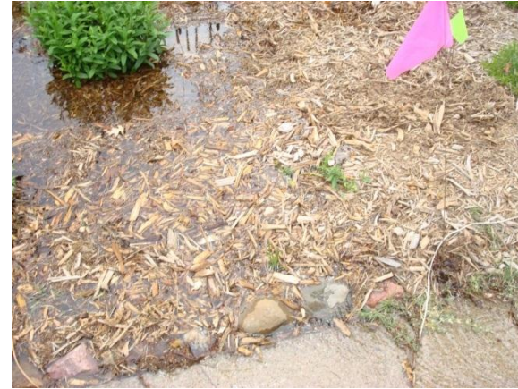
Figure 42. Inundated garden showing widespread outflow onto driveway (designed outflow structure is on opposite side of garden).
