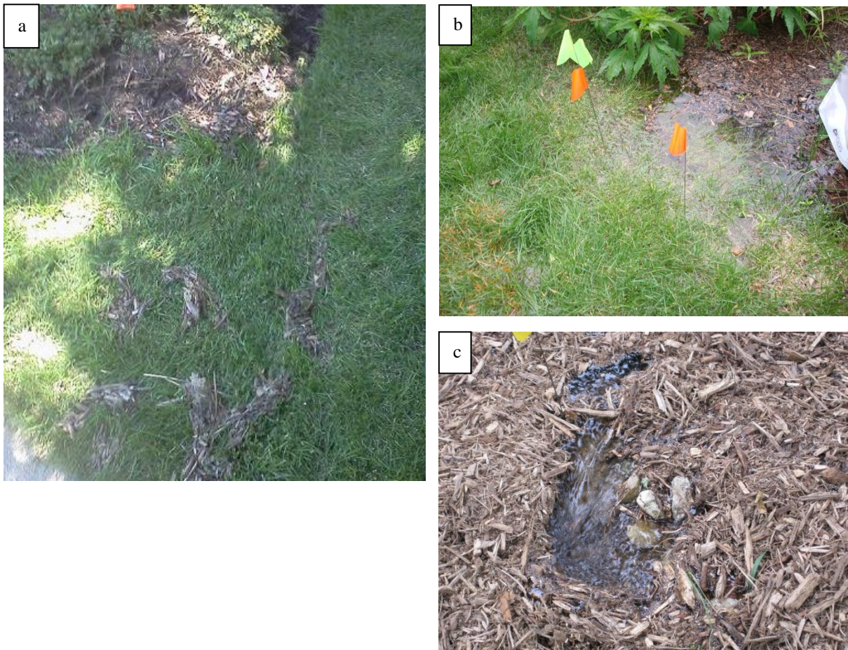
Figure 24. Photographs of failed overflow structures. (a) Outflow is at a low spot of the berm. (b) Lack of overflow structure. (c) Erosion of berm
