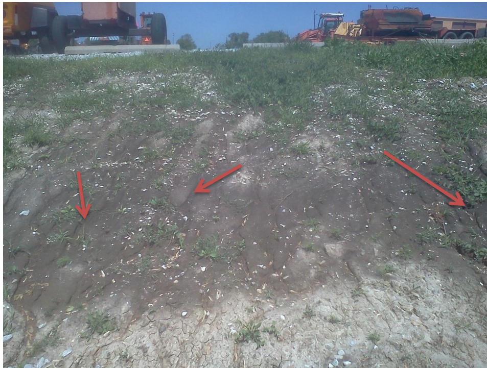
Figure 2.20 Filter trench side slope rills
