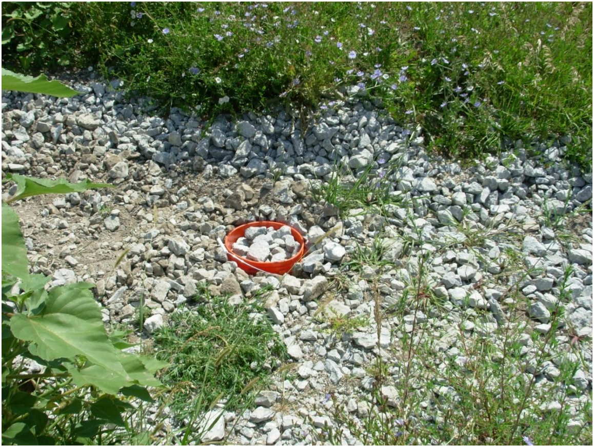
Figure B.12 Sediment bucket in infiltration trench
