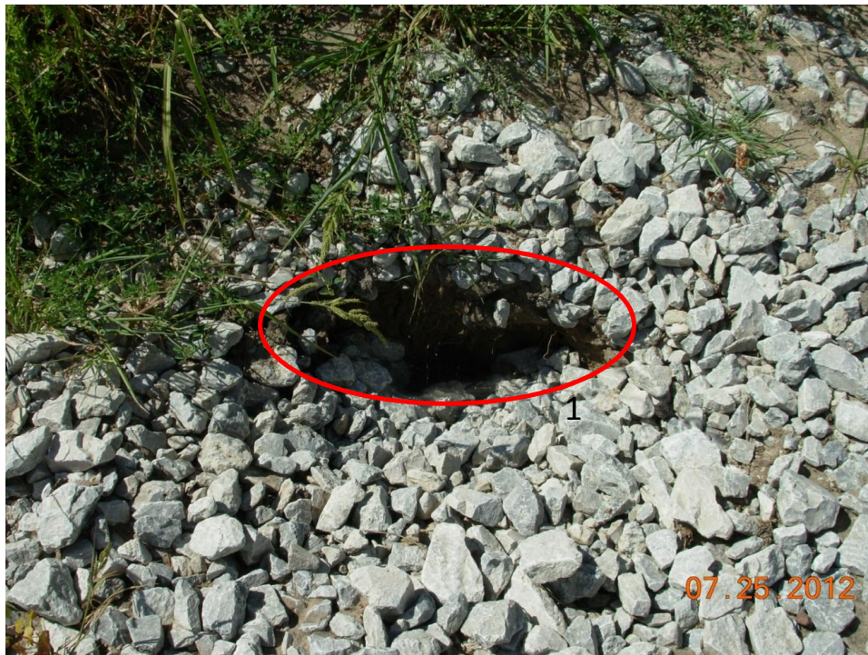
Figure 2.25 Filter trench undermining hole along trench
