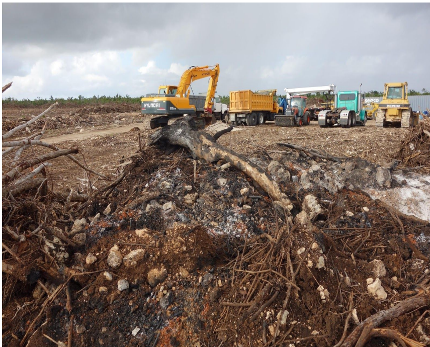
Photo 6. Excavation of the airport in its current position in December 2017. Large excavation equipment can be seen in the background. Vegetation, including rare and endangered species were piled and burned as shown in the foreground.
