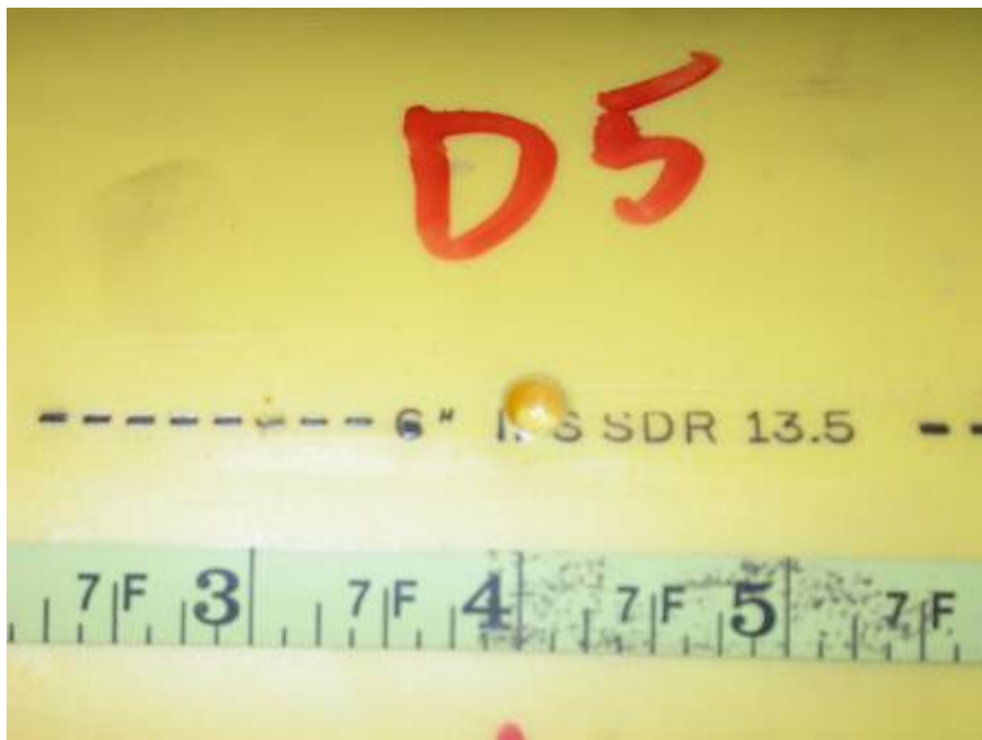
Figure 5-7. Defect D10 (D5)
