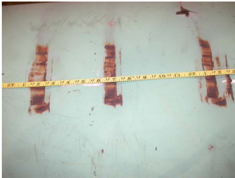
Figure 19. Example Mechanical Damage Defect from Pipe Sample 1
