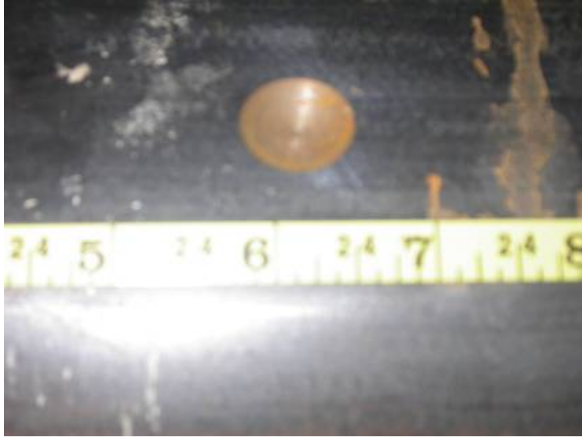
Figure 2-40. Defect P3-19 (Defect 12)
