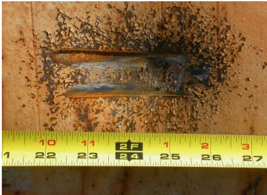
Figure 3-13. Defect D6 (Dent with Gouge; Not Part of Benchmarking)
