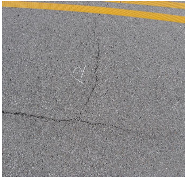
Figure 5.3 Observed multi-crack joint
