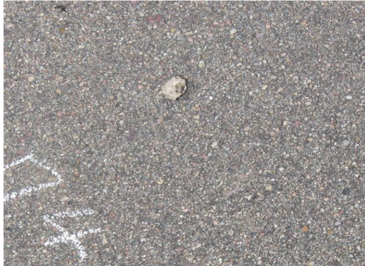
Figure 5.5 Observed Surface Void
