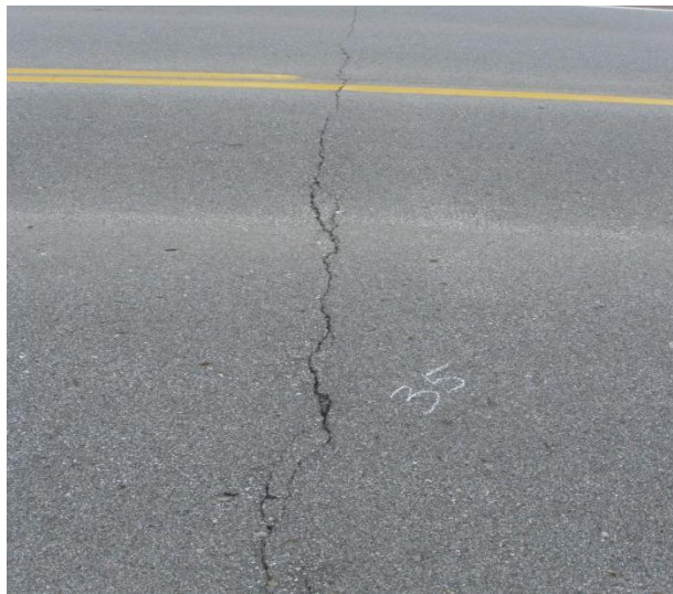
Figure 5.2 Observed Transverse Crack
