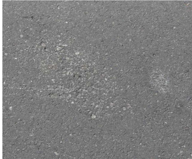
Figure 5.4 Observed Material Segregation
