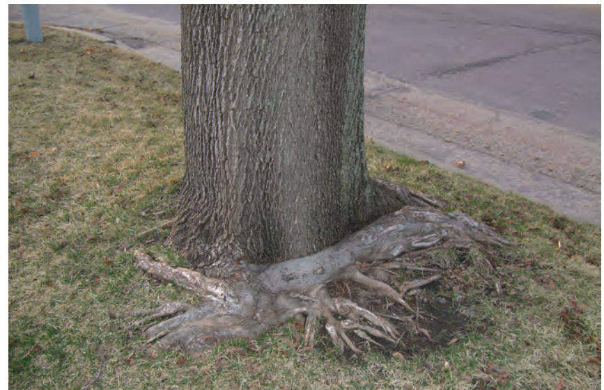
Figure 7. If the entire trunk is encircled by a girdling root, reject the plant.
