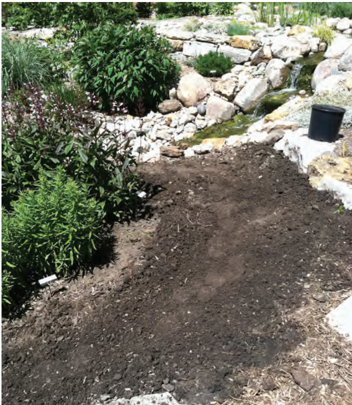
Figure 5. Site preparation in older neighborhoods may be as simple as removing existing vegetation and tilling or raking lightly to reestablish good drainage.
