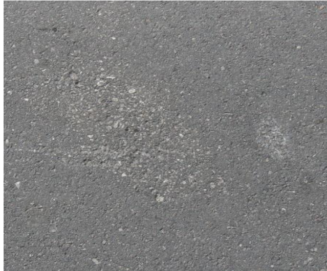
Figure 5.4 Observed Material Segregation
