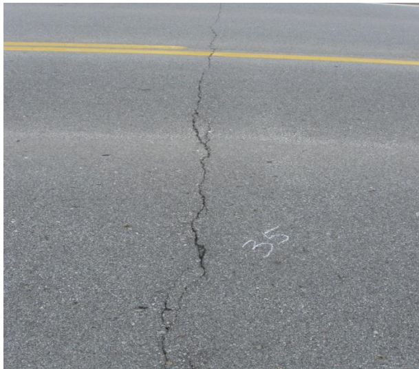
Figure 5.2 Observed Transverse Crack
