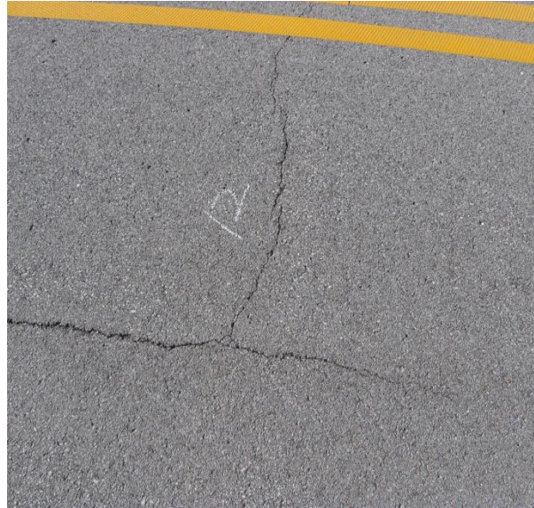
Figure 5.3 Observed Multi-Crack Joint
