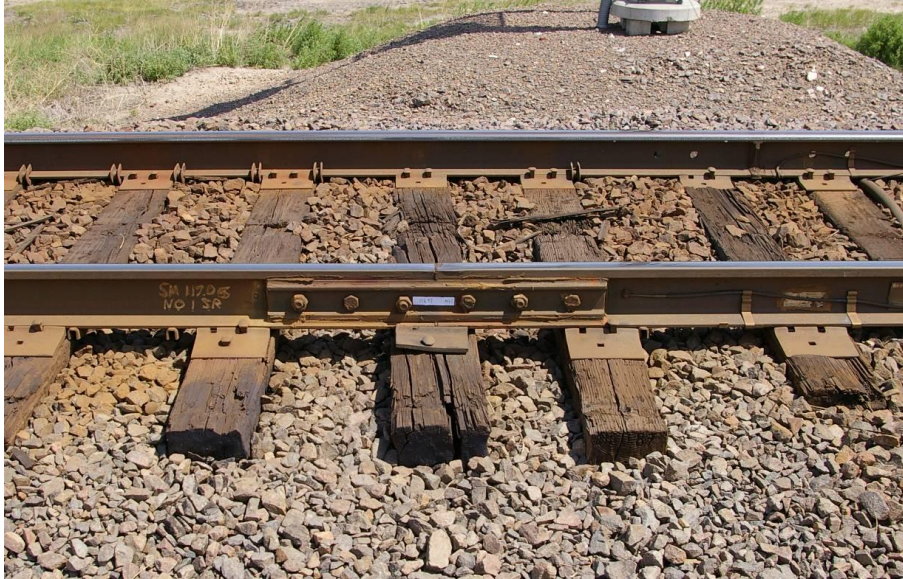
Figure 3-18. Failing insulated joint at site A (Lu, 2008).
