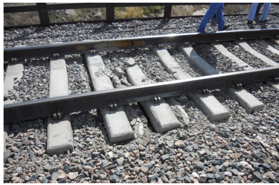
Figure 3-20. Broken ties at site B.
