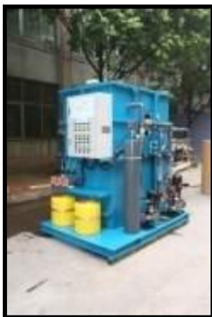
Figure 17: Ultra Filtration (NalSUF) System (Source: Nalco, 2009)
