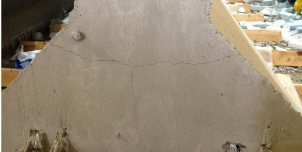
Figure 4.38 End zone cracking at the south end
