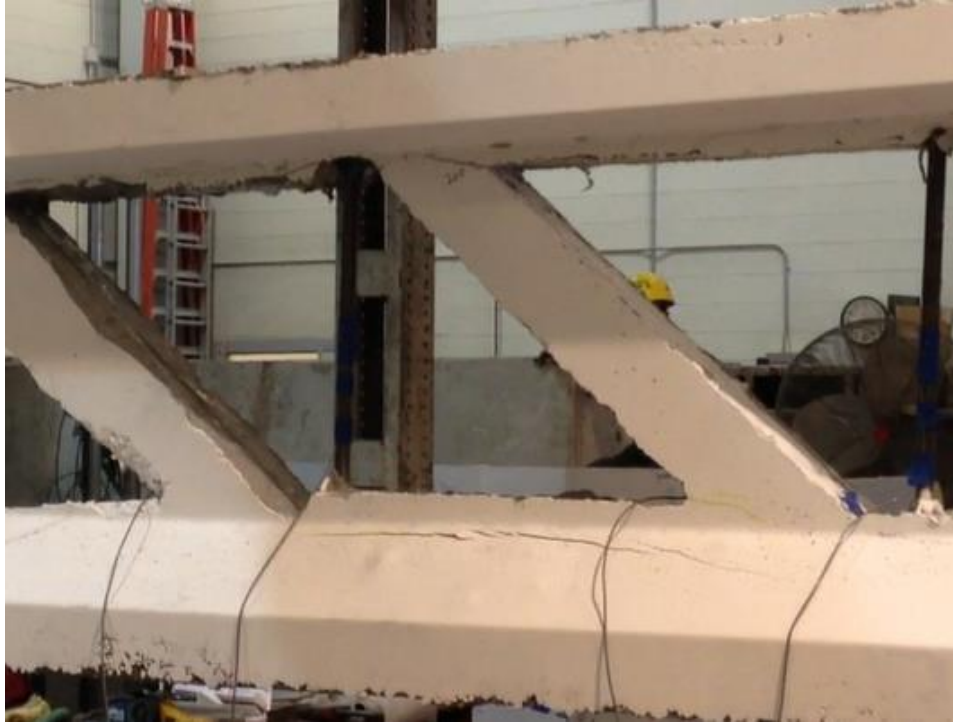
Figure 4.48 Excessive cracking before failure
