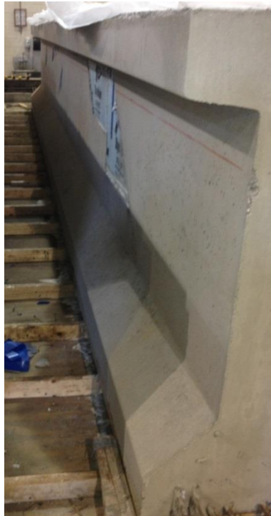
Figure 4.32 The side of the truss after moving the steel form (View is South to North)
