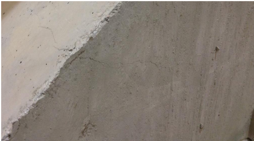
Figure 4.39 End zone cracking at the north end
