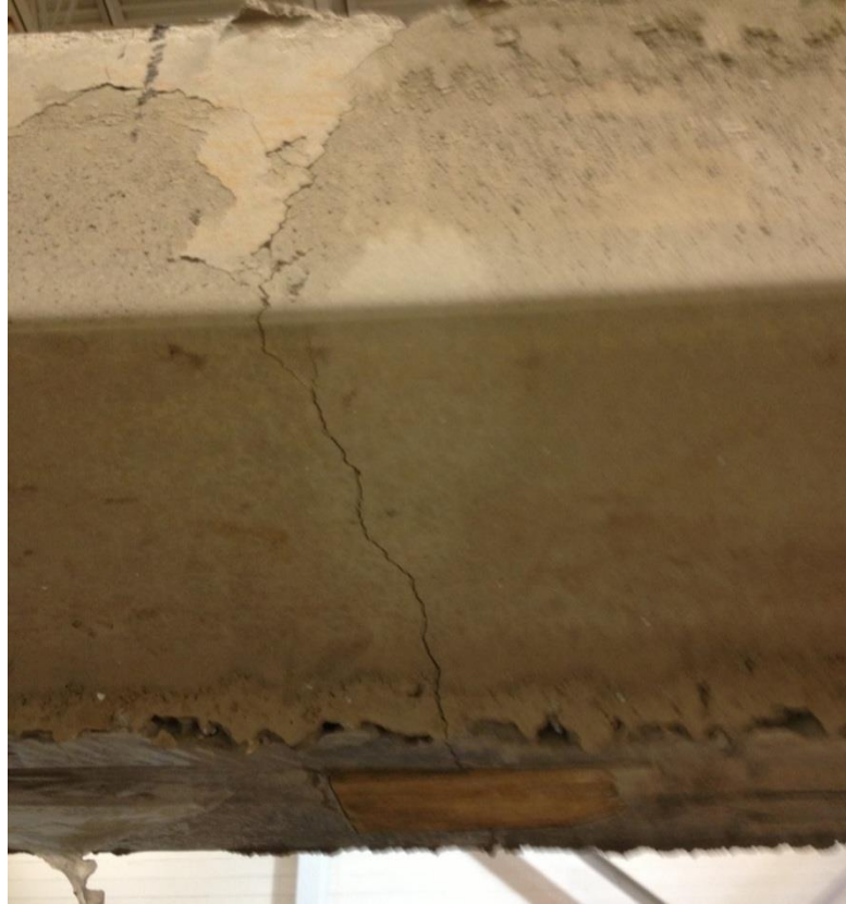
Figure 4.40 Shrinkage cracking where a 2x4 timber piece was left
