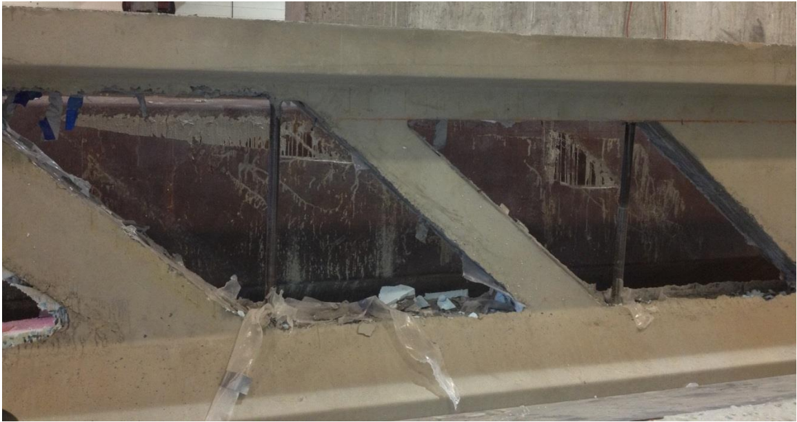
Figure 4.37 Some irregularity that occurred in the truss diagonal and vertical members and locations of block-outs
