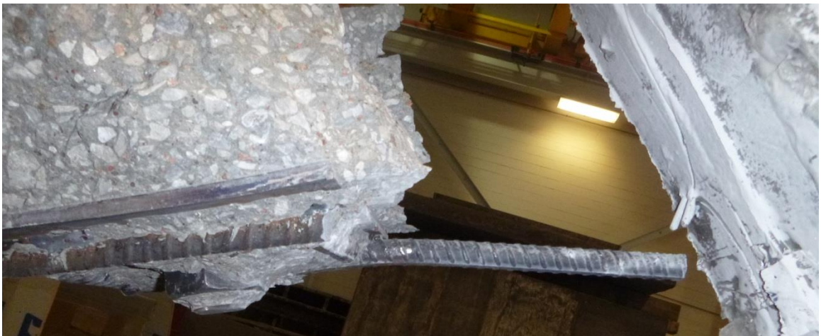
Figure 4.51 The failure of the anchoring bars (one in shear while the other pullout)
