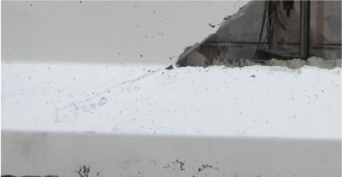
Figure 4.45 Cracking extents vs. loading points for the north diagonal to web connection
