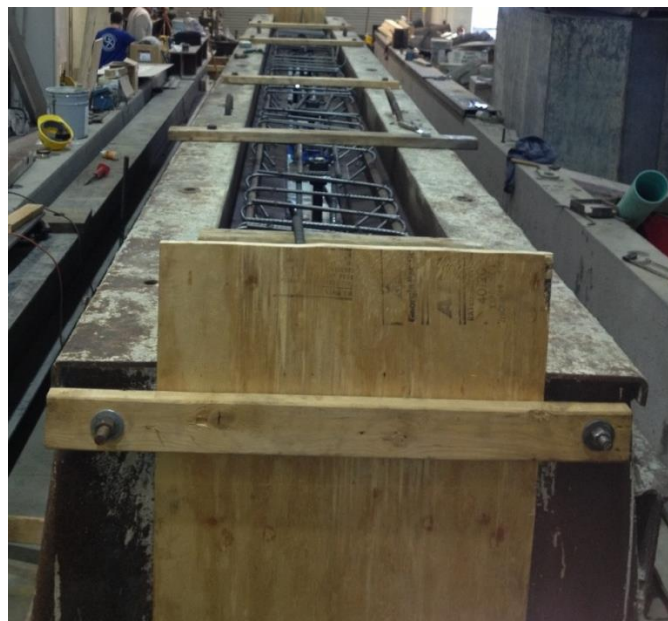
Figure 4.26 The form after adding the top flange reinforcements and adding ties at the top
