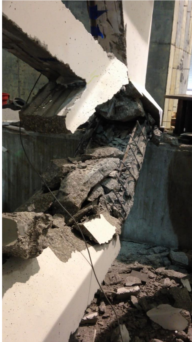
Figure 4.52 Location of failure
