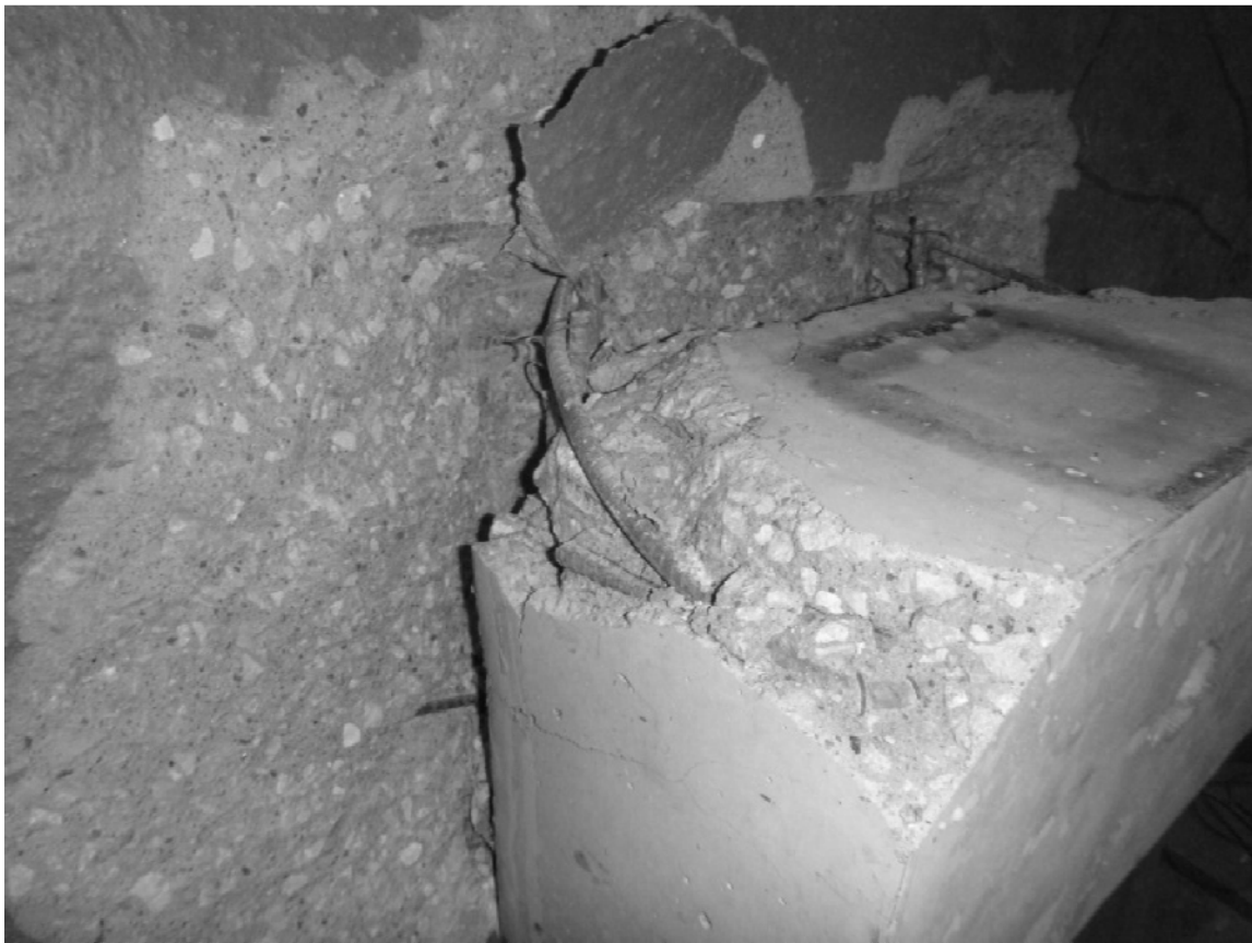
Figure 4-18: Bent stirrups followed by concrete breakout in specimen A5
