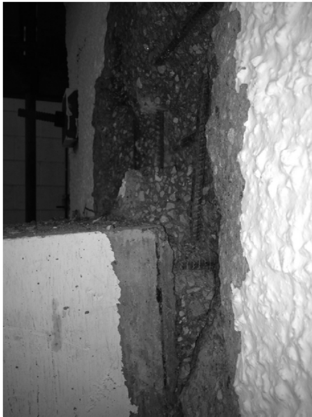
Figure 4-9: Cause of failure for specimen A1, concrete breakout
