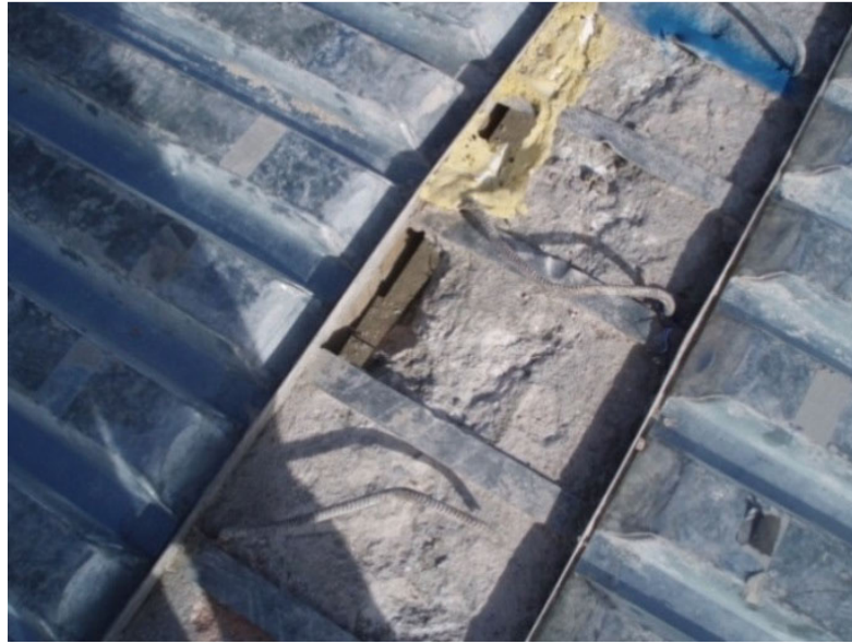
FIGURE 3-23: DAMAGED SHEAR CONNECTORS AND TOP FLANGE OF THE GIRDER
