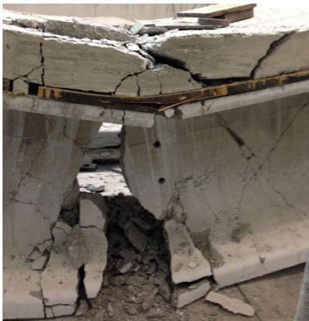
FIGURE 6-33: FAILURE MODE OF FULL FLANGE GIRDER
