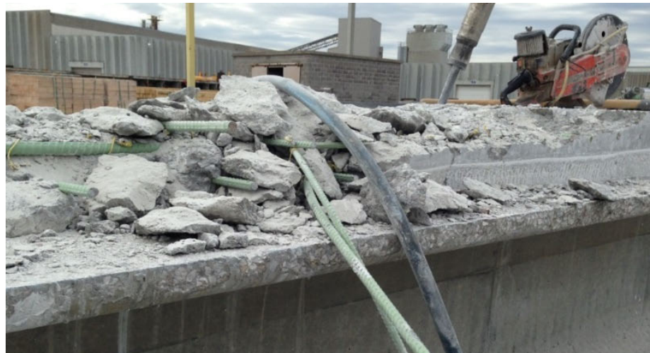
FIGURE 6-16: DAMAGED FLANGE FROM VIBRATION OF 90LB JACK HAMMER
