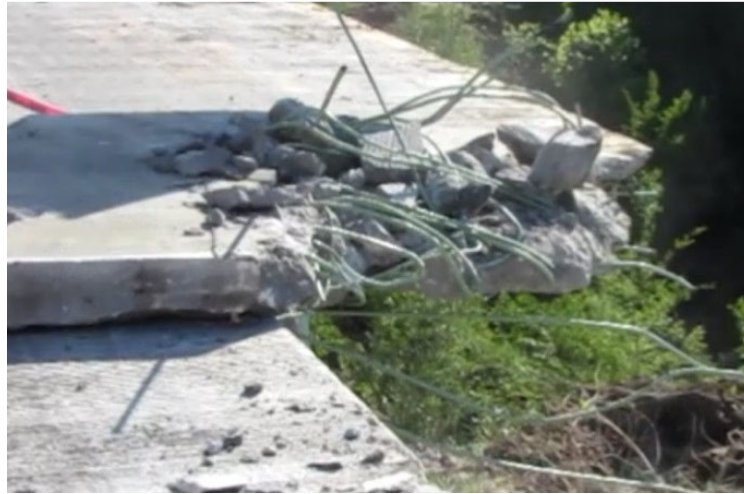
FIGURE 3-13: PART OF THE DECK THAT WAS PEELED OFF
