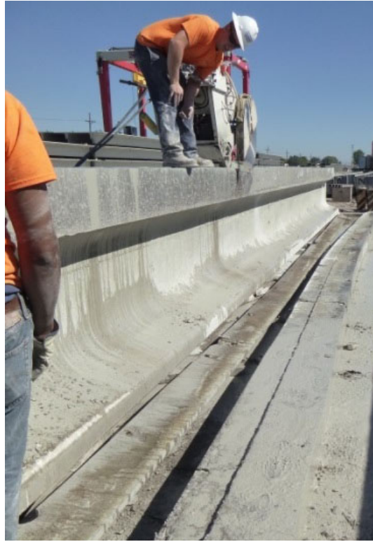
FIGURE 6-10: SEPERATION OF DECK AND FLANGE AFTER FALLING DOWN
