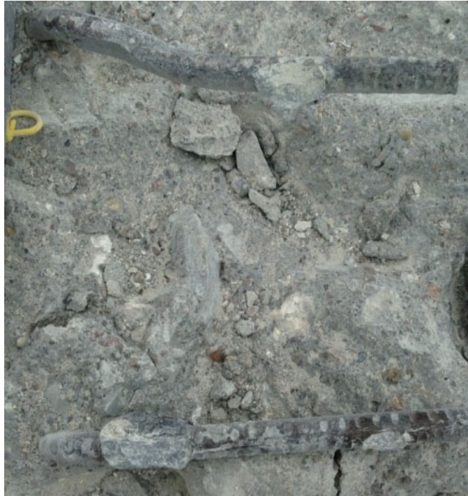
FIGURE 6-17: DAMAGED STIRRUP LEGS
