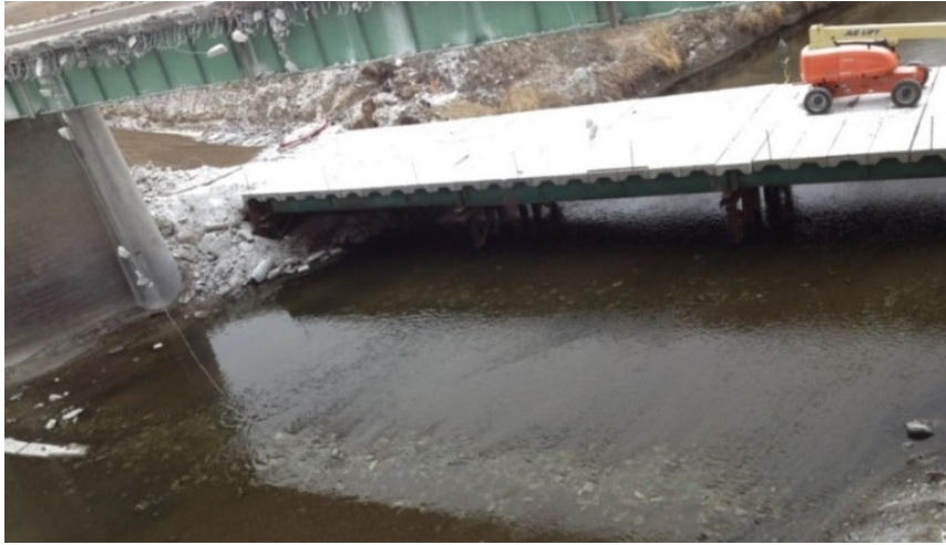
FIGURE 3-27: CONCRETE PIECES FELL TO THE WATERWAY UNDERNEATH
