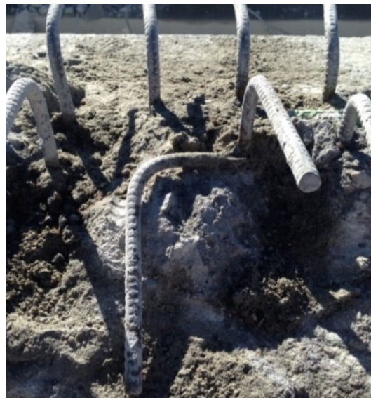
FIGURE 6-23: BROKEN STIRRUP LEG
