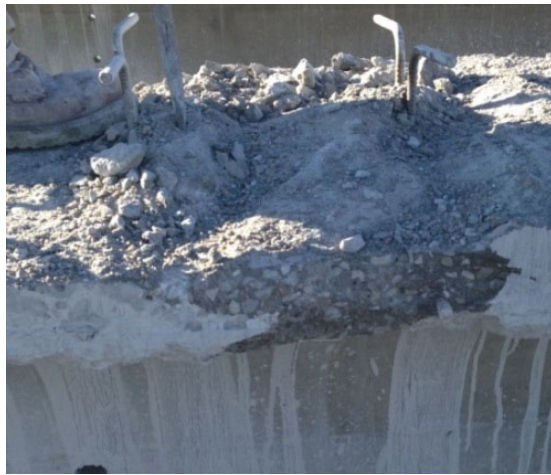
FIGURE 6-22: DAMAGED FLANGE ON GIRDER #2
