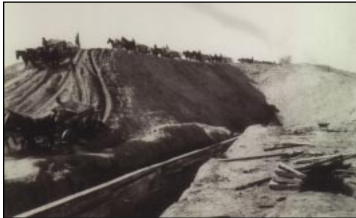
Muscle and determination helped build U.S. Bureau of Reclamation irrigation projects. Here, men and horses haul backfill material for sluicing into a cut-off trench at Minatare Dam in October, 1913. Additional copies of the October, 2002 Water Current giving the history of Bureau projects in Nebraska and eastern Wyoming are available free from the UNL Water Center (USBR photo).
