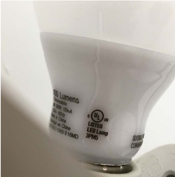
Figure 3.9 High Efficacy Lighting Verification
