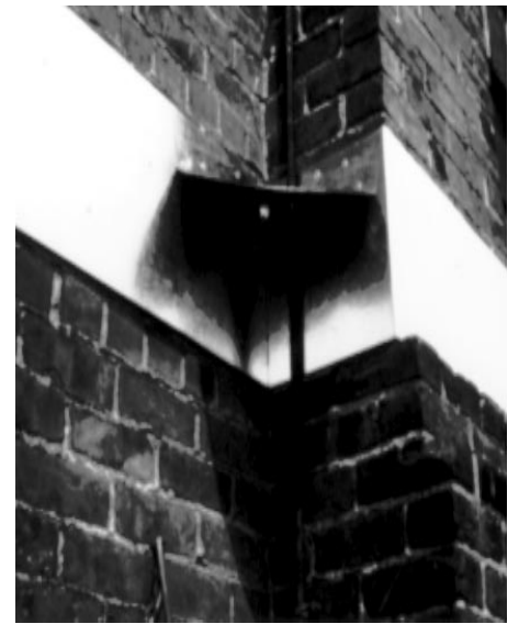
Fig. 20. Sheet metal band attached to outside walls to prevent rodent climbing. Band should be 14 to 18 inches wide and 30 inches above where a rodent can jump from.
