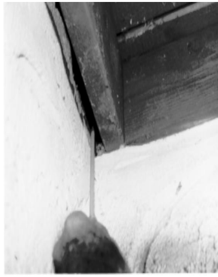
Fig. 4b. Gap (3/4 x 26 inch) between wall covering and framing at roof joint, allowing rats and mice easy access.
