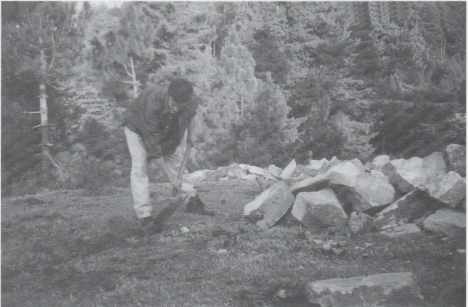
Owen Joiner starting to dig the foundations of the captive breeding station at Shinkiari.
