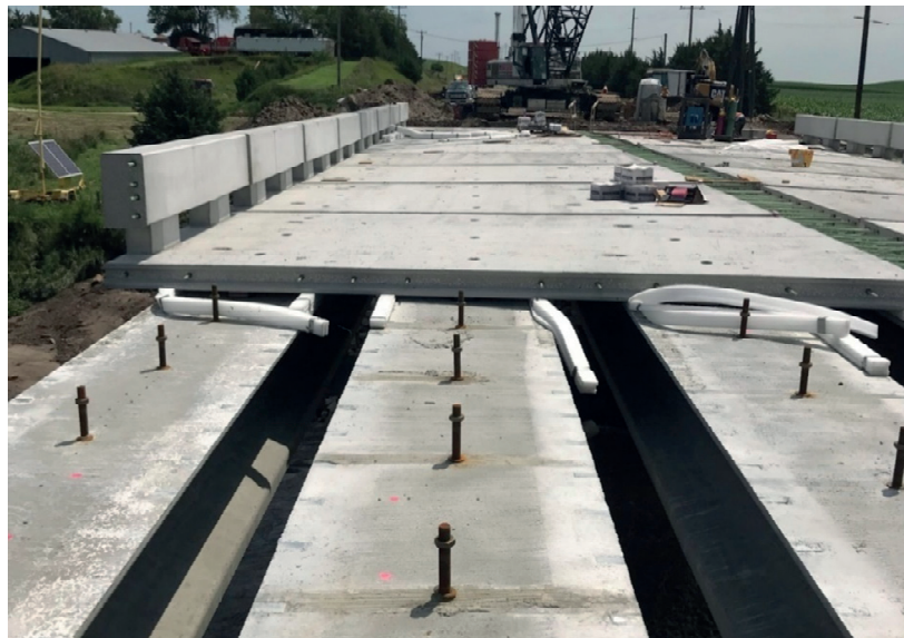
Figure 1.2. Precast Concrete Deck-to-Girder Connections using threaded rods and HSS-formed shear pockets used in Kearney East Bypass Project (top) and Belden-Laurel Bridge Project (bottom)
