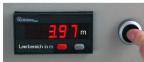
Figure 2.4 A display unit at the silo displays the empty space (in meters) or the filling level in percentage. (Dimetex, 2004)
