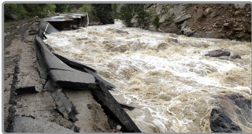
Above: Destroyed road in Boulder, CO - courtesy Daily Camera
