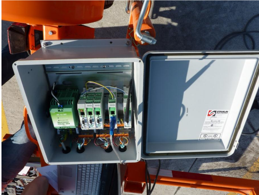
Figure 3.12 Portable sensor pole cabinet
