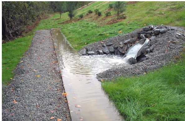
Figure 12.10 Improper entry to level spreader (Winston et al. 2010)
