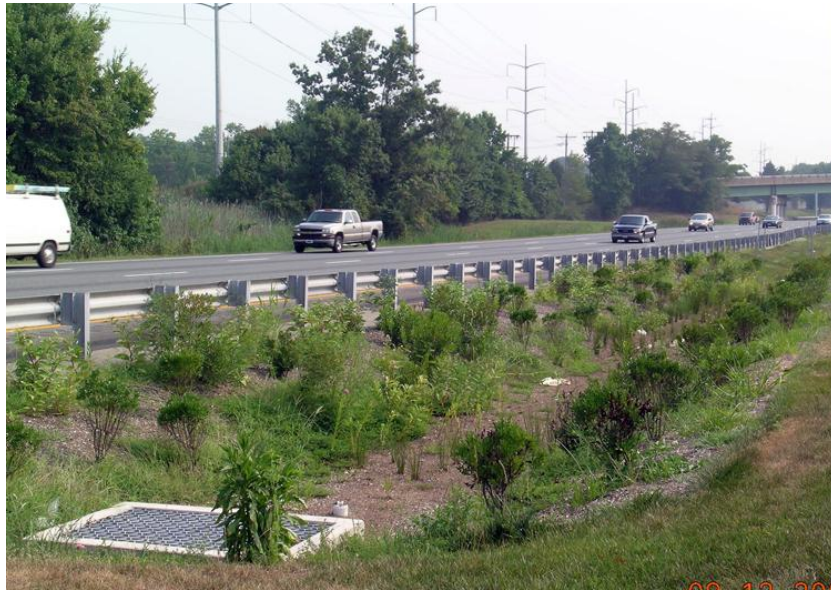
Figure 12.3 Highway median bioretention in Delaware (DelDOT 2012)
