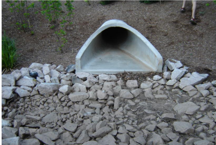
Figure 13 Properly utilized forebay (NCDENR 2007)
