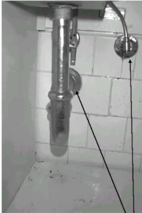
No gaps between pipes and wall
