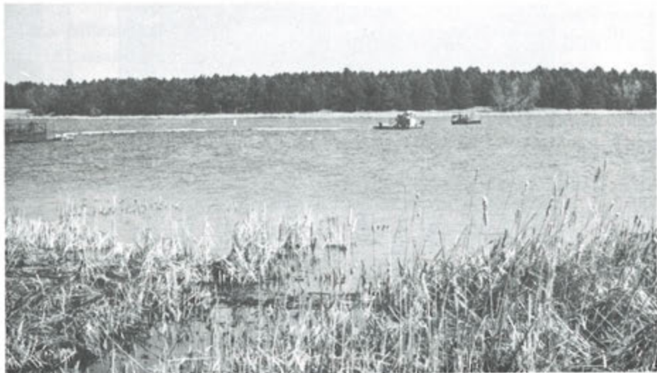
Dredging at Smith Lake SRA was 50% complete with removal of 65,500 cubic yards of material in this Aquatic Habitat project.
