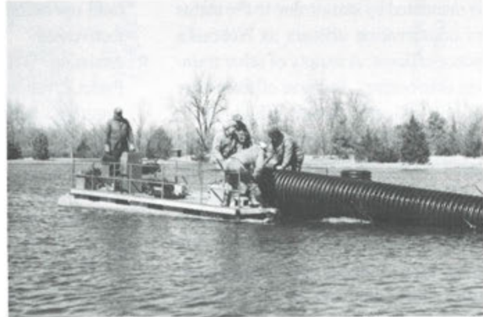
Aerator installed on trout lake at Two Rivers SRA was specially designed by agency engineer, Dwight Hanson.
