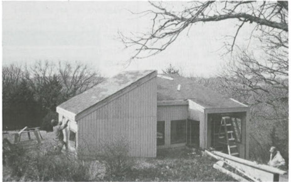
Division carpenters are remodeling and improving the seven Wild Turkey Cabins at Platte River State Park. After 15 years of use new roofs, siding and insulation were needed, along with painting inside and out. Heating and air conditioning were also installed.
