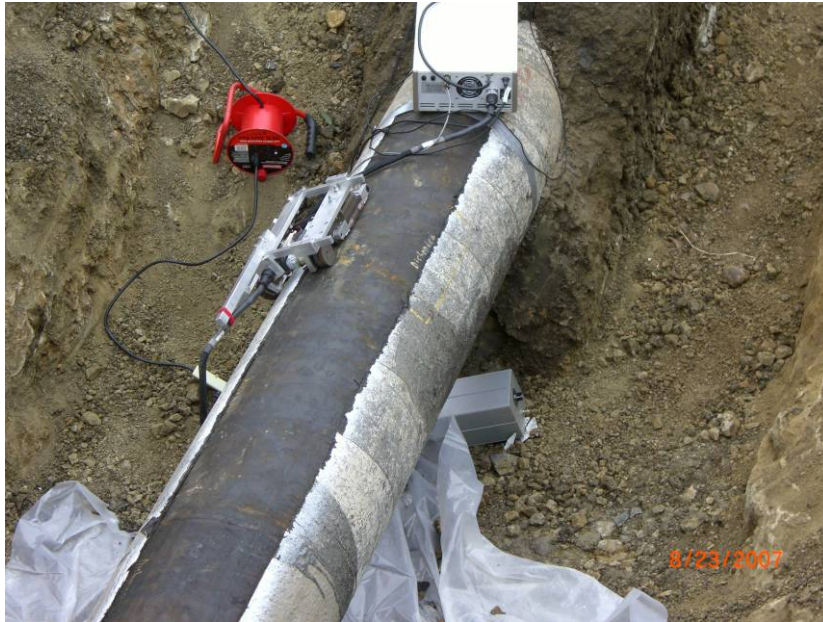
Figure 3: Field demonstration at an ECDA dig on a 20" asphalt coated pipe. The scanner is shown half on the 1/4" coating and half on the bare pipe. The inspection instrument is on the pipe at the top of the photo.
