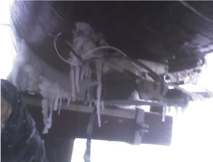
Figure 2: EMAT CIRC Scanner with icicles scanning the bottom of the 34” oil transit line in Prudhoe Bay Alaska.
