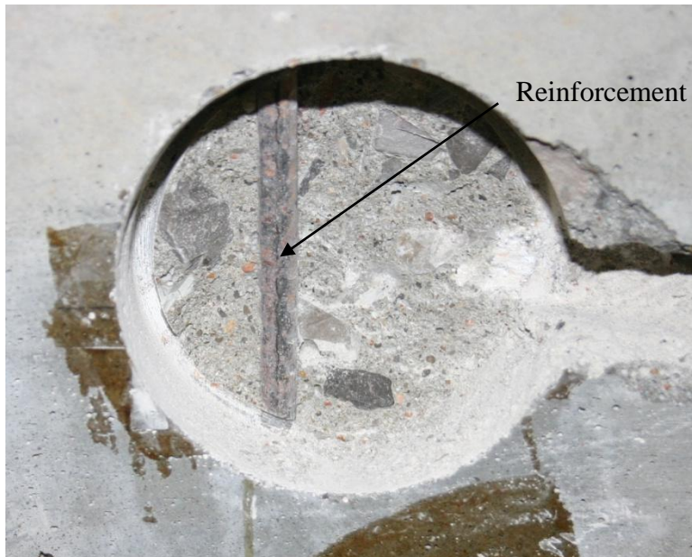
Figure 7.1 Reinforcement Affecting Strain Relief on the Surface of the Core
