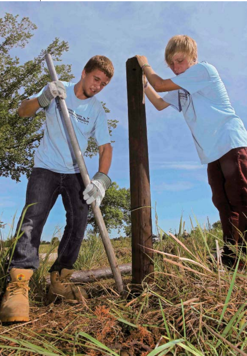
As part of the Nebraska Youth Conservation Program, Tyler Yates (left) and Nick Shelor, both of Lincoln, set a post while installing a new fence at Pawnee SRA last summer.
