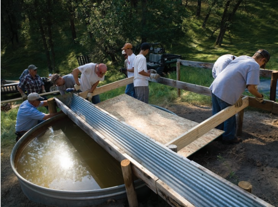
Water catchments funnel rainfall into a tank, that is then used by a variety of wildlife species. Members of Scout Troop 201 out of Chadron replace parts of a catchment on Metcalf Wildlife Management Area located 12 miles north of Hay Springs.
