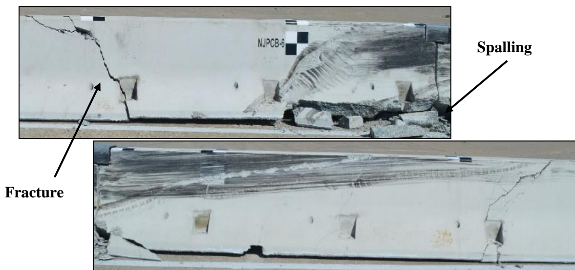
Figure 39. Barrier Damage – Barrier 4 (Top) and Barrier 5 (Bottom)
