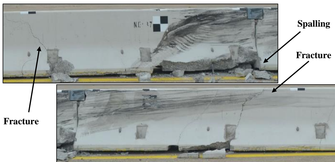
Figure 43. Barrier Damage – Barrier 4 (Top) and Barrier 5 (Bottom)
