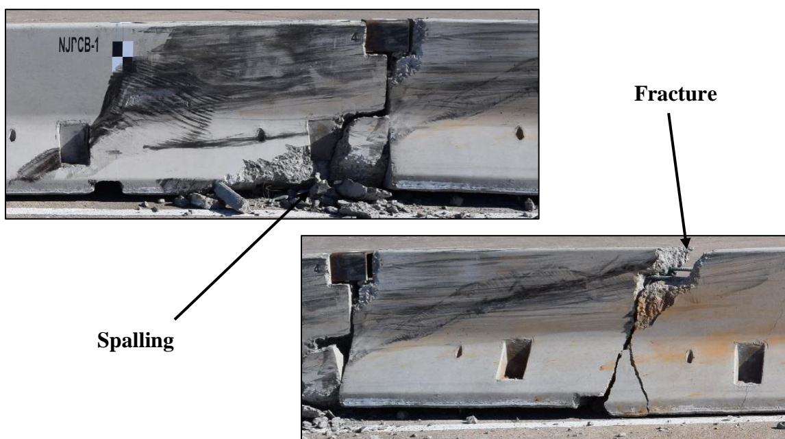
Figure 19. Barrier Damage – Barrier 4 (Top) and Barrier 5 (Bottom)
