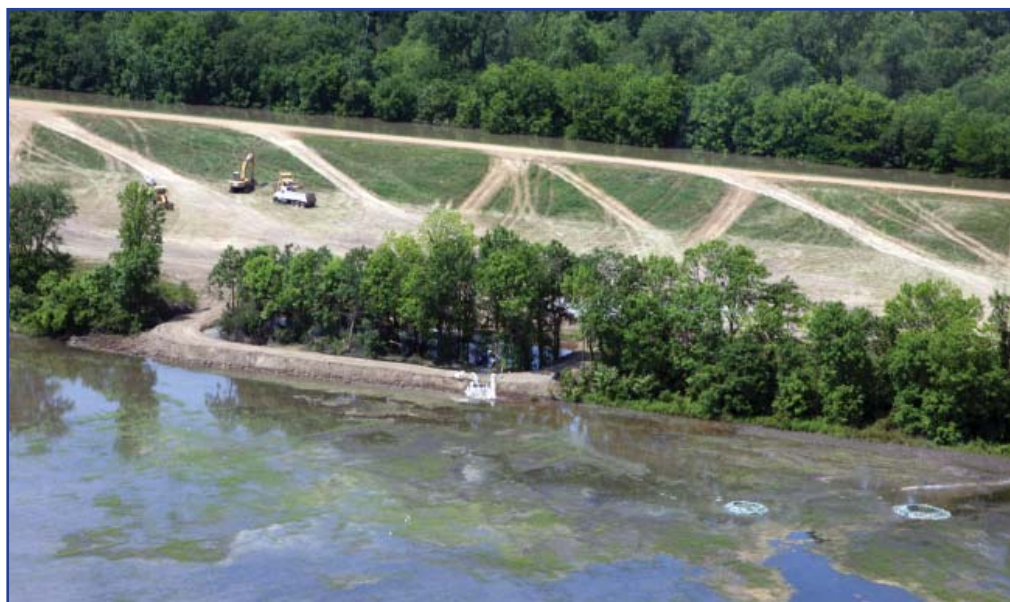
The completed water berm at Francis, Miss. Note the additional sand boil rings in the foreground and the river stage in the background.
