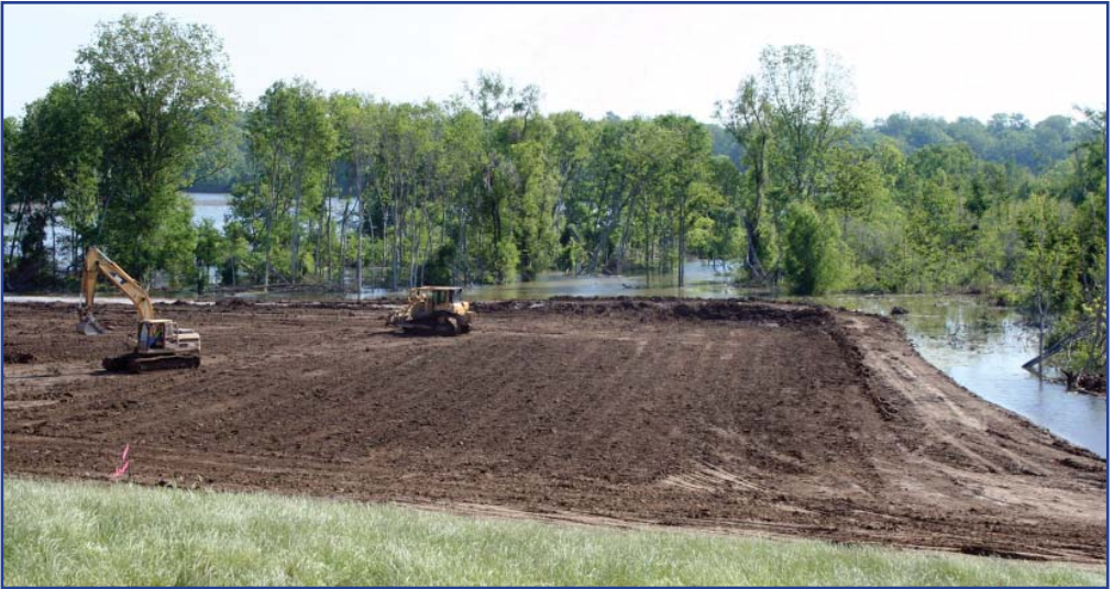
The clay cap nears completion at Buck Chute as water from Eagle Lake continues to rise.
