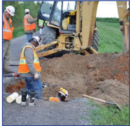
Memphis Engineer District work crews unearth the access wells at the Birds Point-New Madrid floodway fuseplug levee.
