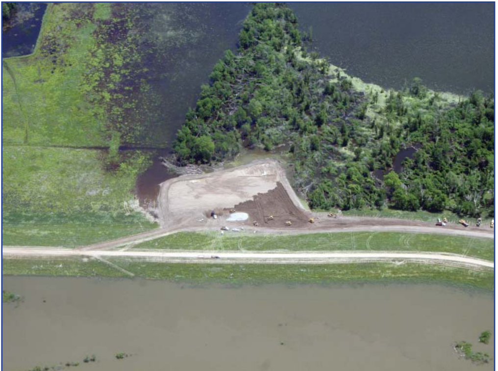
The hired-labor crew begins placing the clay cap over the sand fill as water from Eagle Lake climbs higher against the earthen berm.
