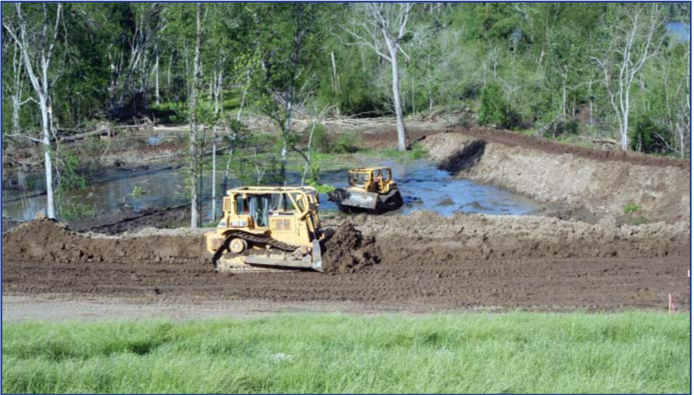
Hired-labor crews construct the earthen berm around Buck Chute, while continuing to clear the area.
