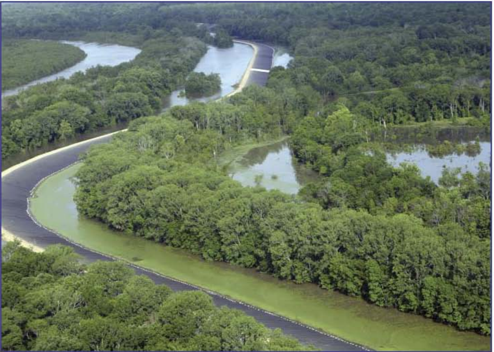
The river encroaches upon the gravel road at the crown of the armored Yazoo backwater levee. Note the trapped interior drainage to the right of the levee.
