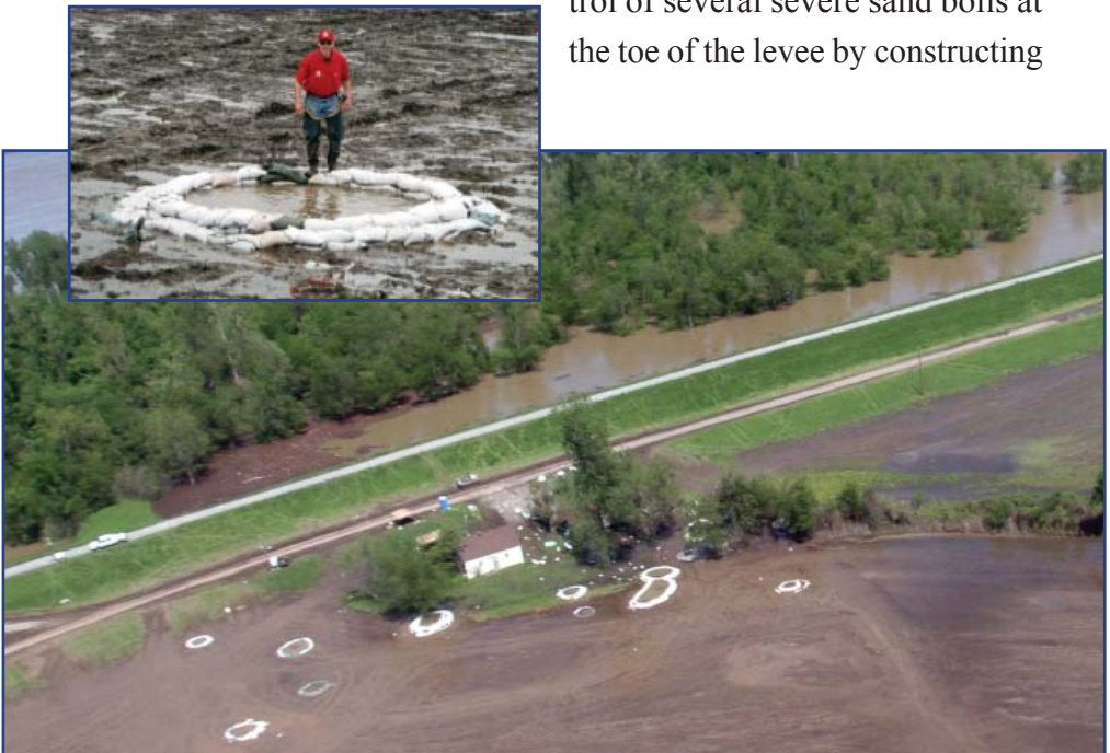
Sand boil rings near the toe of the levee surround a home in Fulton County. Inset: Darian Chasteen stands next to a sand boil ring in muddy Fulton County, Tennessee.
