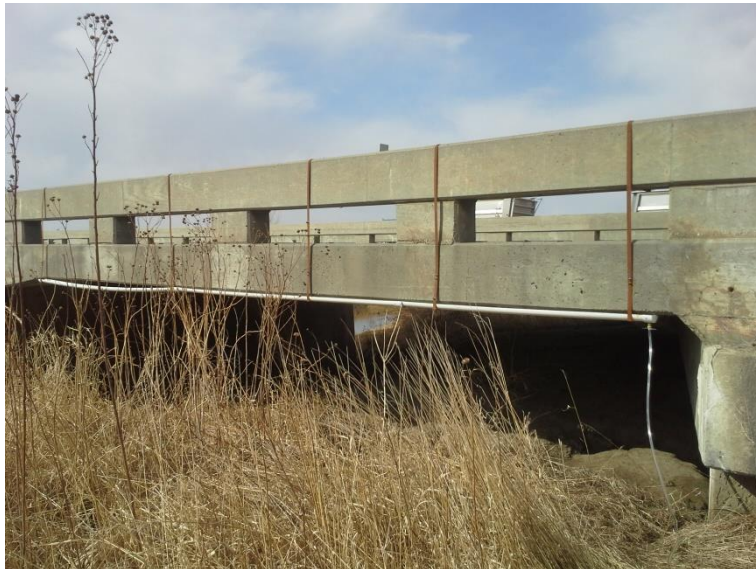
Figure 2.2 Bridge gutter system installed at Highway 77 over Rock Creek near Ceresco
