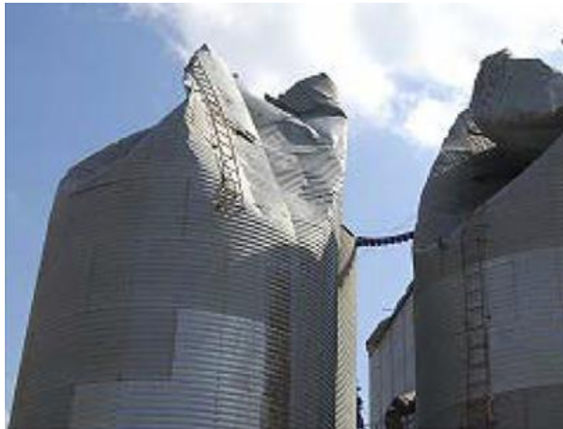
Fig. 2.5 Severe buckling of the cylindrical shells (Kikitsu and Sarkar 2015)
