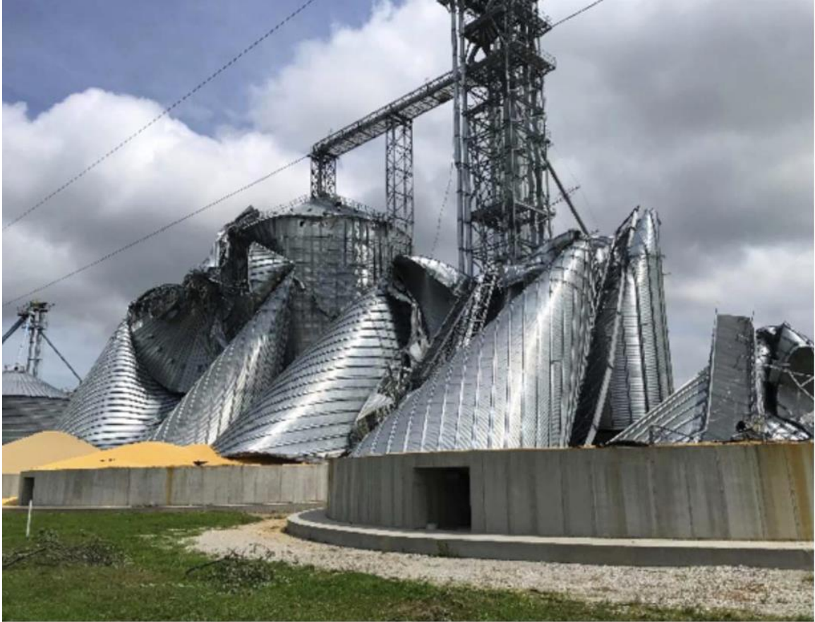
Fig. 2.6 Grain Bin Damage from August 10 derecho (Shouse et al. 2021)
