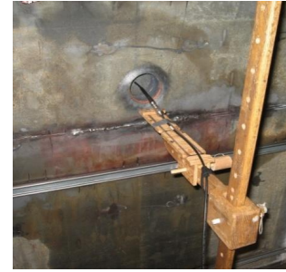
Fig. 4 Monopole antenna extended into concrete dome from inside the shelter
