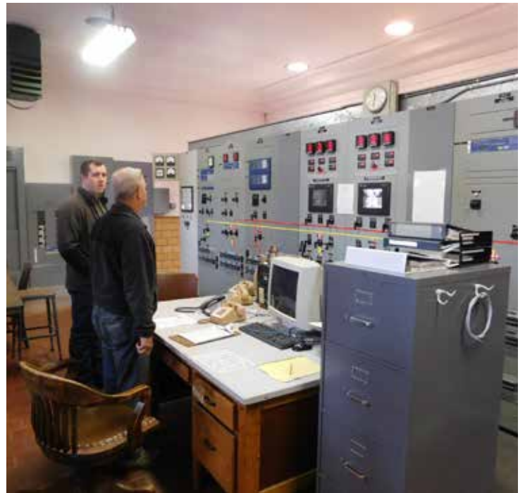
Ben Beckman and Jeff Buettner look over the control panel for a hydro-power station at Johnson Lake.
