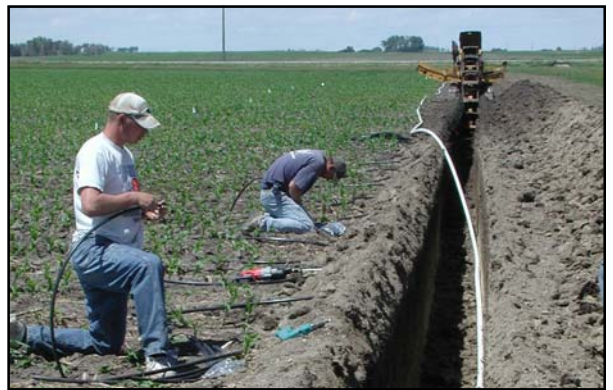
Installing subsurface drip irrigation lines at UNL's South Central Agricultural Laboratory near Clay Center (photo: Suat Irmak).
