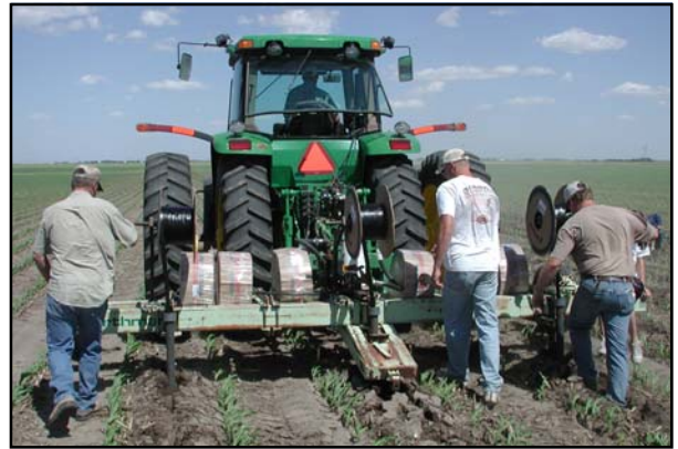
Spools of plastic subsurface irrigation line, or drip tape, are buried about a foot below the surface of this field at UNL's South Central Agricultural laboratory near Clay Center (photo: Suat Irmak).
