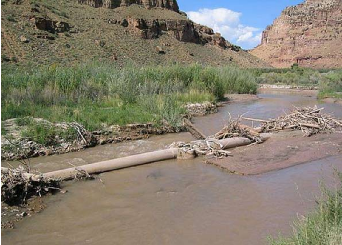
Figure 10. Lateral migration of this stream channel during high water excavated a section of pipeline under the floodplain that was several feet shallower than at the original stream crossing.
