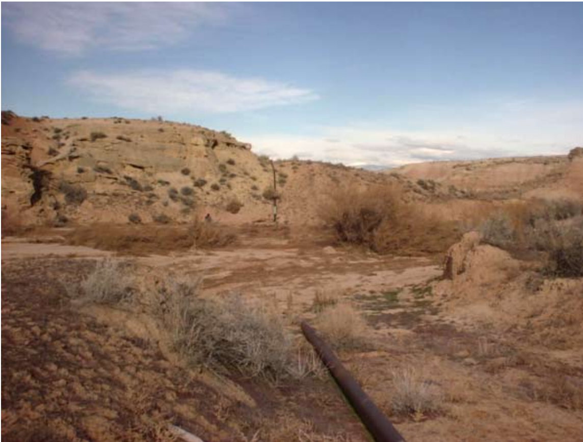
Figure 6. Channel degradation or scour during flash-flood events may expose buried pipelines, resulting in costly breaks.
