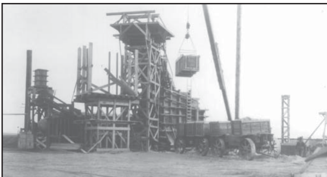
Construction of Minatare Dam in western Nebraska, like many early Reclamation projects, included having to elevate skips containing gravel into a hopper that screened the gravel. This photo dates to November, 1912. For perspective, that's little more than seven months after the ocean liner RMS TITANIC struck an iceberg and sank in the North Atlantic (USBR photo).
