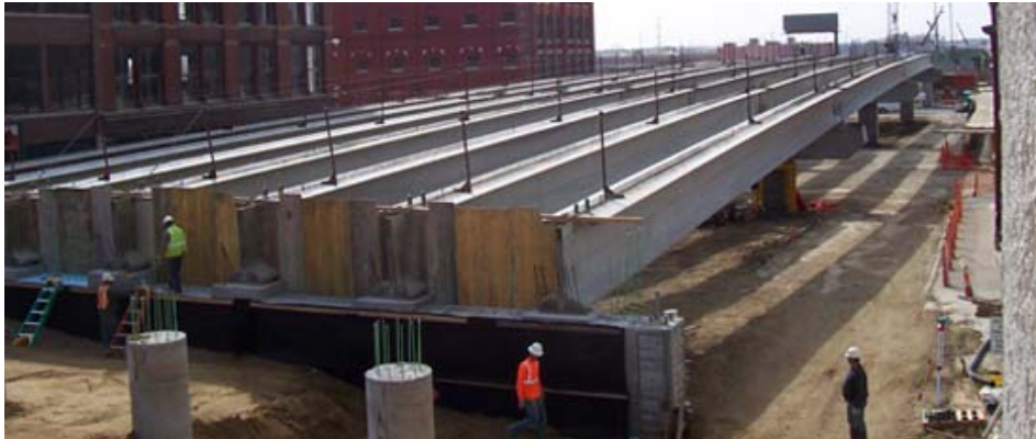
Self-consolidating concrete with a compressive strength of 12,000 psi (83 MPa) was used in the beams of the Harris Overpass, Lincoln, NE.
