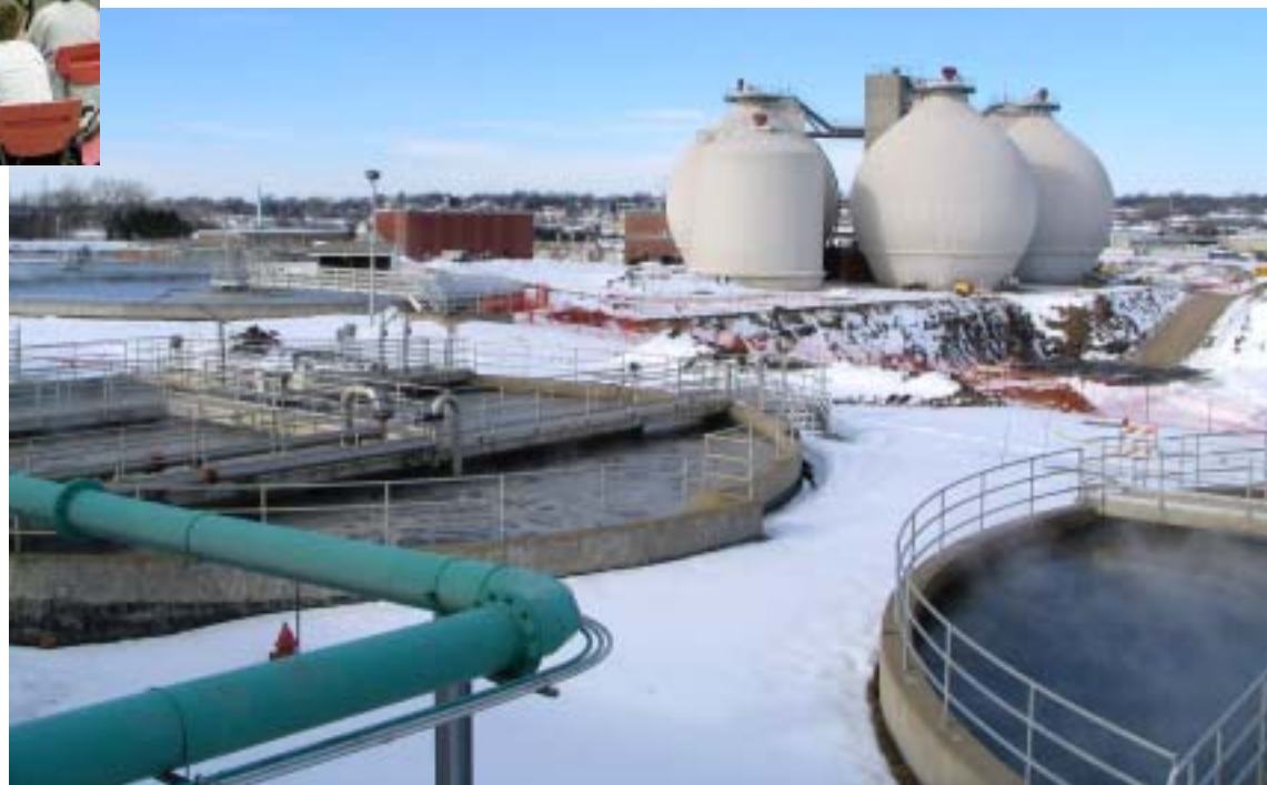
The Theresa Street Wastewater Facility, southwest of 27th and Cornhusker cleans wastewater and produces biosolids 24 hours, 7 days a week and never shuts down for holidays. This facility is currently undergoing major construction to increase capacity to keep pace with Lincoln's increasing population.
