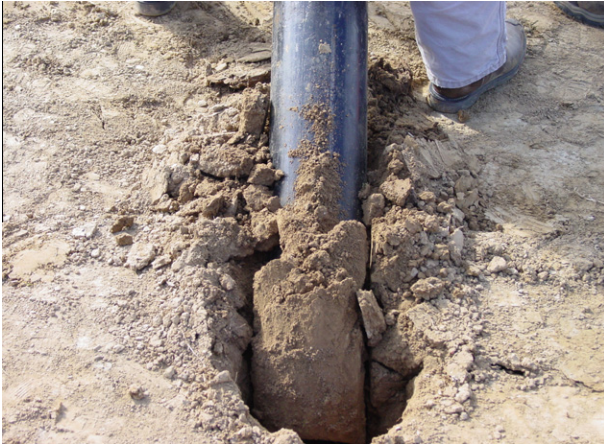
Fig. 5. Posts after failure.
